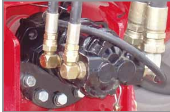
PTO pump installed
